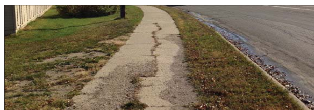
Cracked and uneven sidewalks
